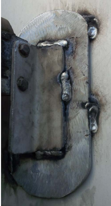
Examples of pads without continuous welds
