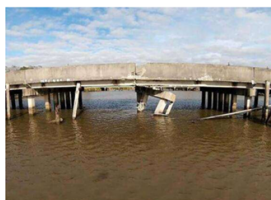
Figure 59: Bayou Ramous Bridge Strike
