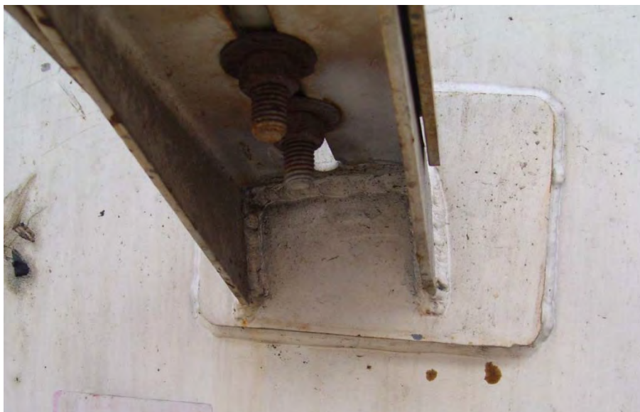
Example of Improper Pad
